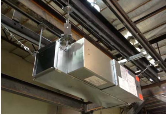
FIGURE 2 – SECTIONS OF 45-DEGREE AND 90-DEGREE BRACKETS WITH 1/2" DIAMETER ALL-THREADED ROD AND 3/16" DIAMETER STEEL CABLING ARE USED TO HANG THE VAV UNITS.
